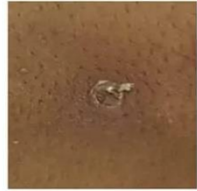
f) partially removed scab
